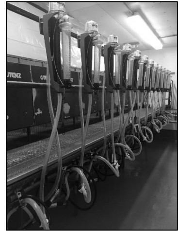
Ready for metering
